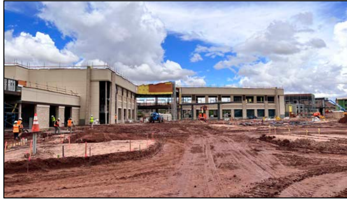
PHOTO: The construction site of the new Sage Memorial Hospital in Ganado, Ariz. on Oct. 4, 2022.
