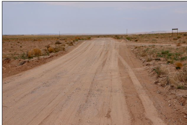
PHOTO: N71 located in Birdsprings, Ariz. on Aug. 12, 2021.
