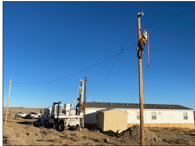
PHOTO: NTUA work crews connect electricity to a home in the community of Naschitti, N.M. on Nov. 28, 2020.
