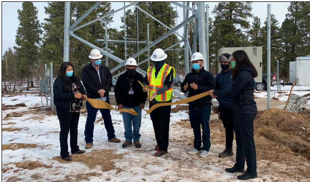
PHOTO: Navajo Nation President Jonathan Nez and NTUA officials celebrate the completion of a new NTUA Choice Wireless tower in Summit East, Ariz. on Dec. 17, 2020.
